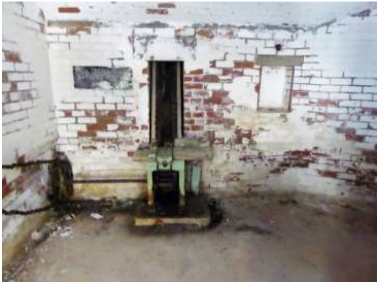
Figure 13 Lentney Battery: the upper and lower ends of an ammunition lift © David Pinder
